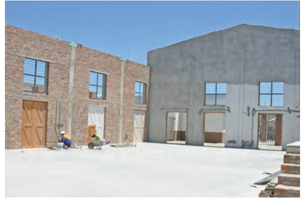
These pictures were taken in the first week of the 2011 school year. The buildings, including the hall, were incomplete and surrounded by a wide expanse of windblown, Cape Flats sand.
